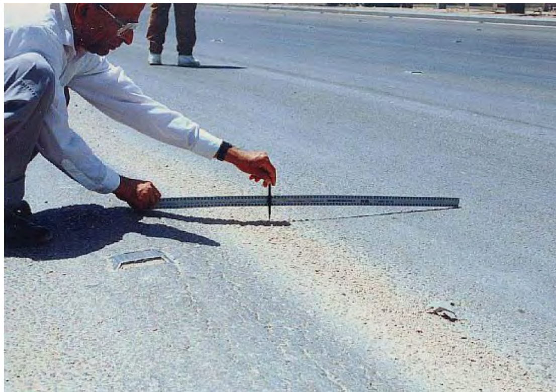
Rutting in Flexible Pavement
