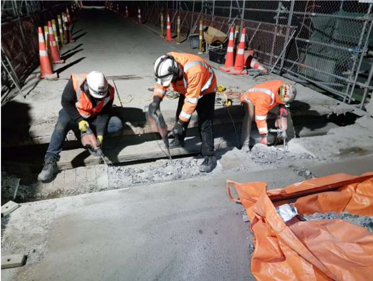
Breakout of headwall at Christchurch end of structure during night closure (Source: Downer NZ)
