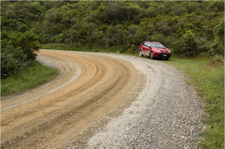
Lake Road at Rosie Bay Abandoned due to accidental grading
